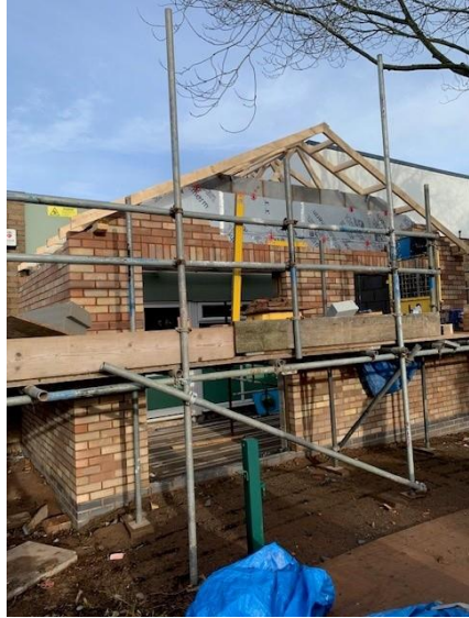
Burley Gate Primary School – Single Story Extension to the front of the school (new Library / Reception Area)
